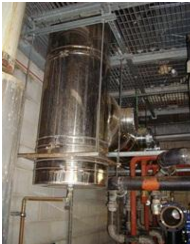
Existing Flue Systems
