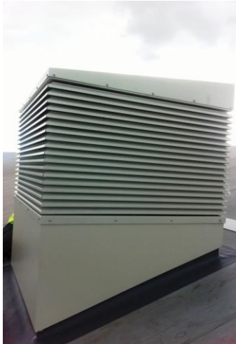
Natural Ventilation Terminals
