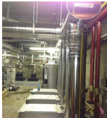
Reay House Boiler Room
