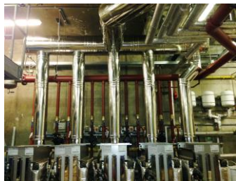
Oak House Boiler Flue System
