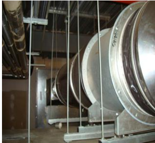
Flue Dilution System
