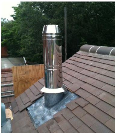
External Flue System
