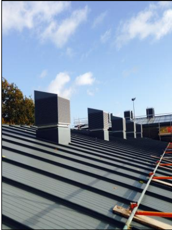
Classroom Ventilation Terminals
