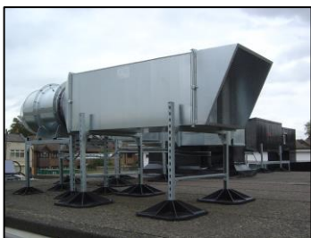
External Supply Air Ductwork
