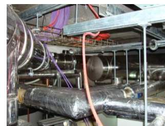
Boiler House – Internal flues
