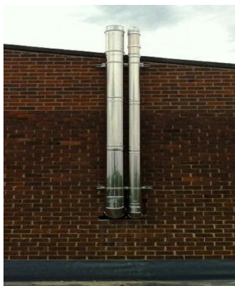
External twin wall flues
