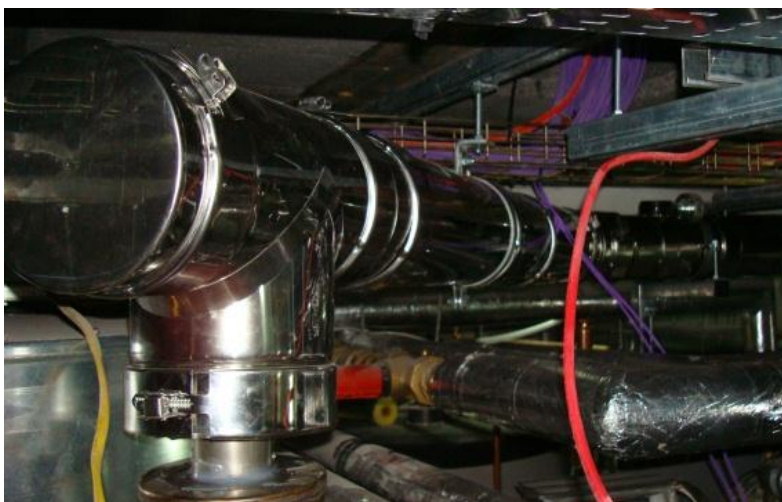
Internal twin wall flues
