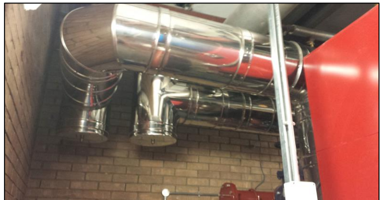
Boiler Room Flues
