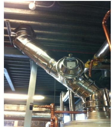
Draft Regulator Fitted
